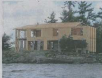
BELOW The basic frame of the main house takes shape. TAYLOR HANNAH ARCHITECT INC.
